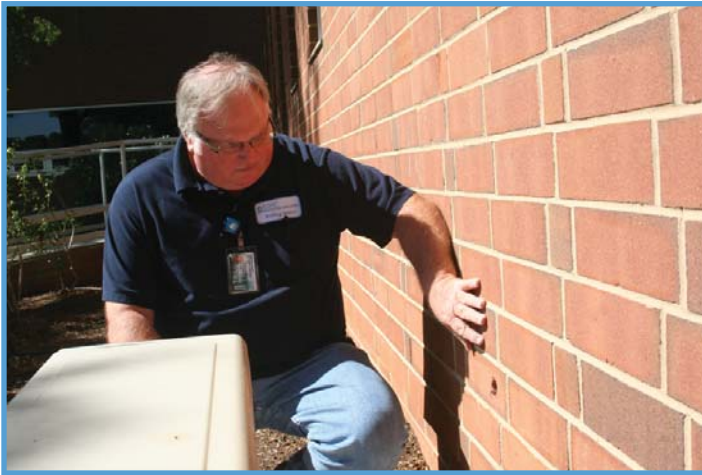
Robert Cooper inspects a campus building to ensure pests have not infiltrated the structure
