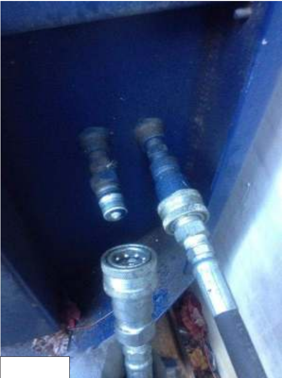
Hydraulic hose unplugged [Figure 10]
