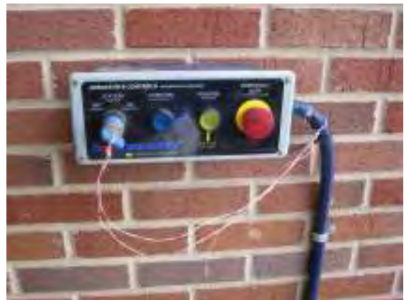
Program to remove keys left in compactors
